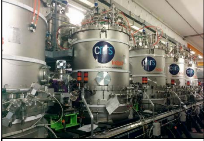
Spiral2 : Integration and test of 7 cryomodules
