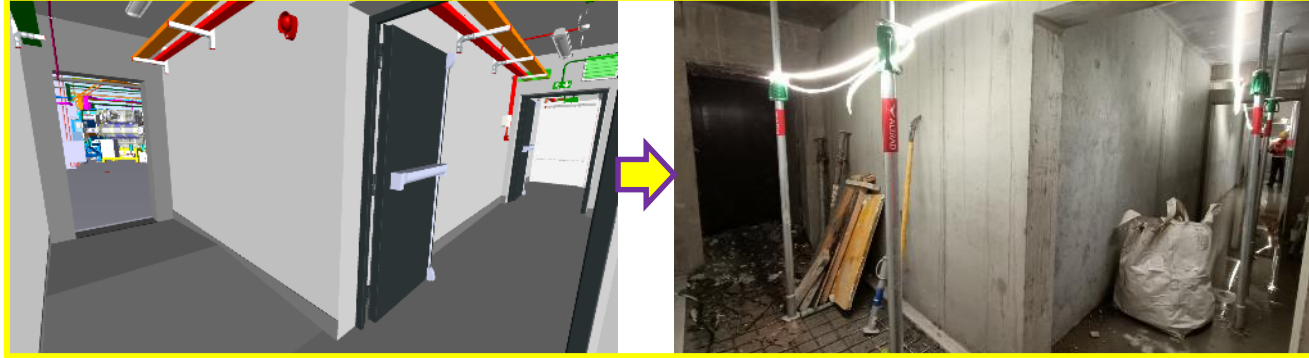
S3/DESIR emergency exit
