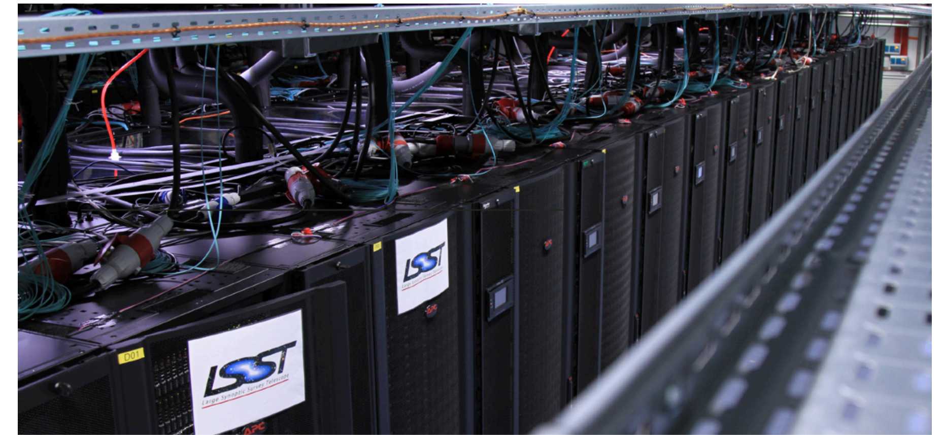
LSST racks at CC-IN2P3
