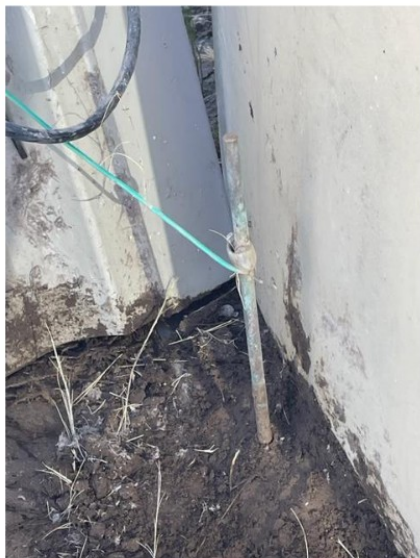
Figure 3: Grounding rod behind the battery box of Saturno.
