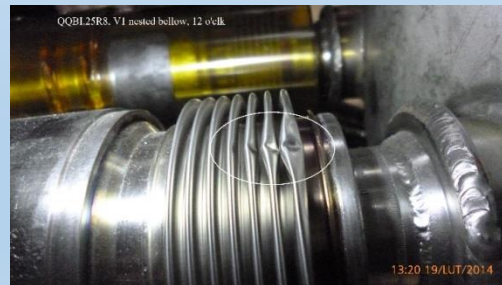
Damage disclosed during QC- ICIT TEAM
