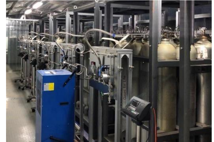
Gas storage system
