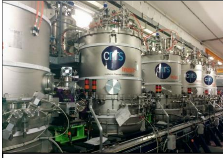
Spiral2 : Integration and test of 7 cryomodules
